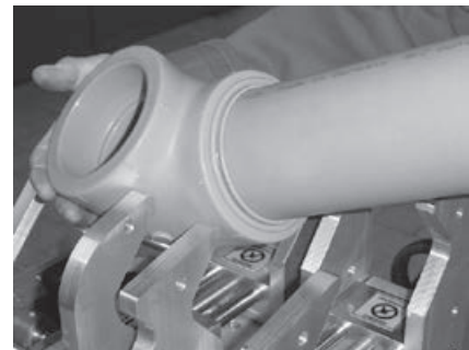
Fig. 12 Remove the welding joint after the end of the cooling time from the clamping jaws
