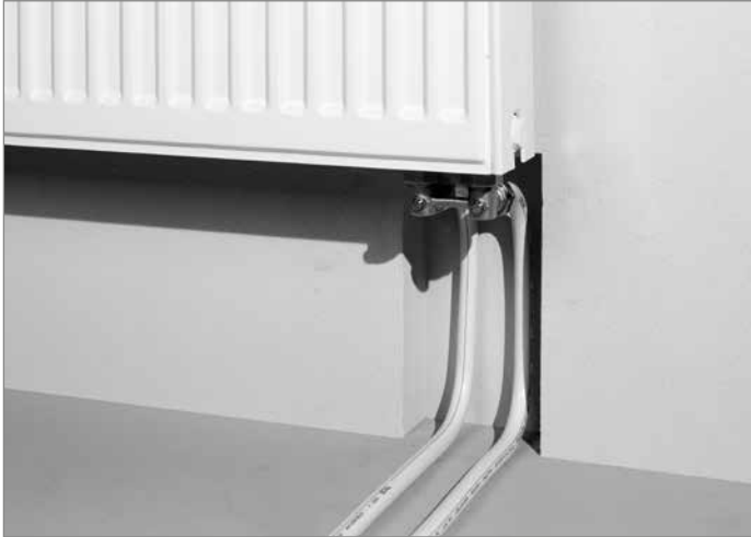
Radiator connection from the wall
